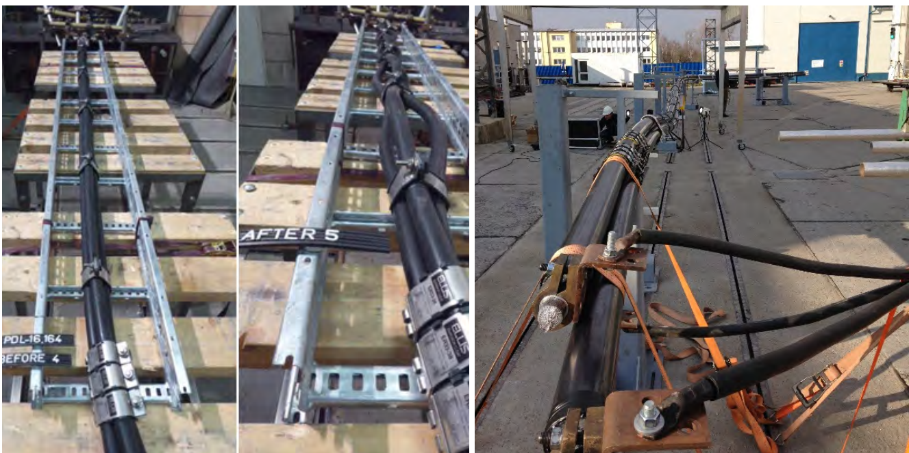
TYPICAL TESTING TO IEC 61914 AND BESPOKE TESTING OF A HV TEST RIG TO A CUSTOMER'S SPECIFICATION.
